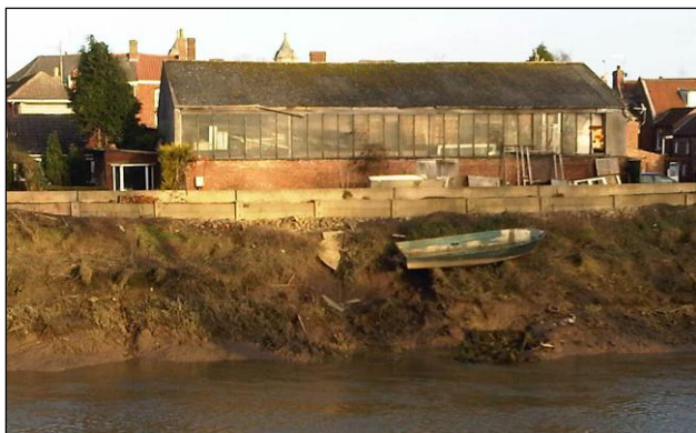
Bank slippage - Boston
