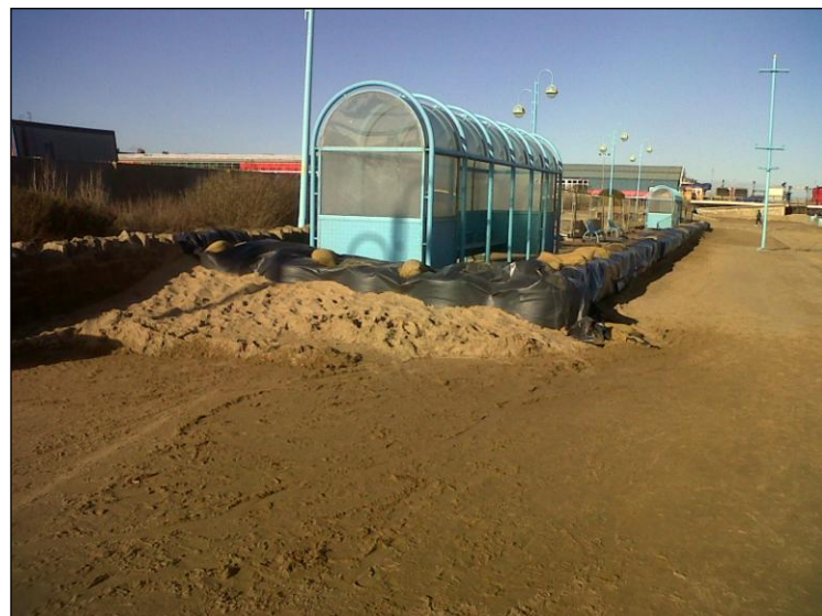
Damage to the flood wall
