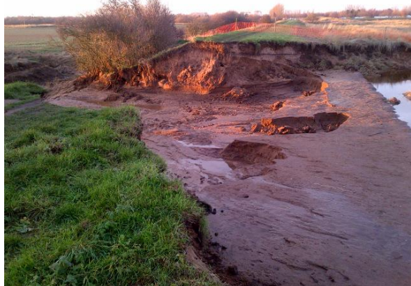
Breach on morning 06.12.13
